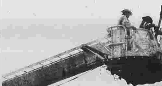
Construction workers on the widening of Vernon Street near the Greenwood Drive intersection.
